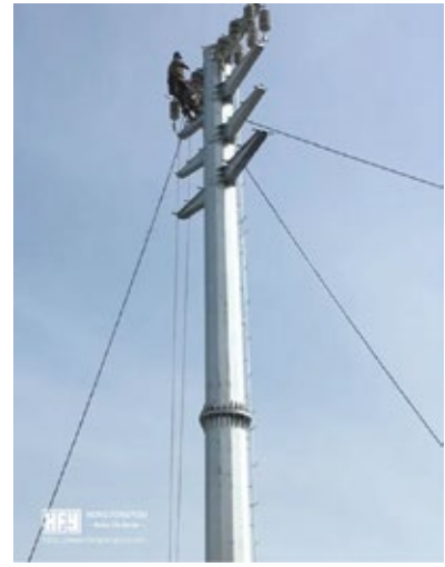
Steel Pole Tower
