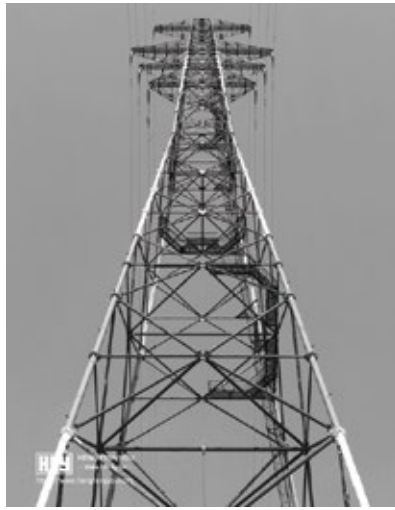
Steel Tubular Tower
