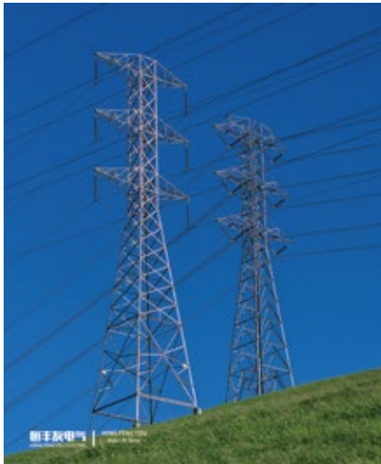
Lattice Steel Tower
